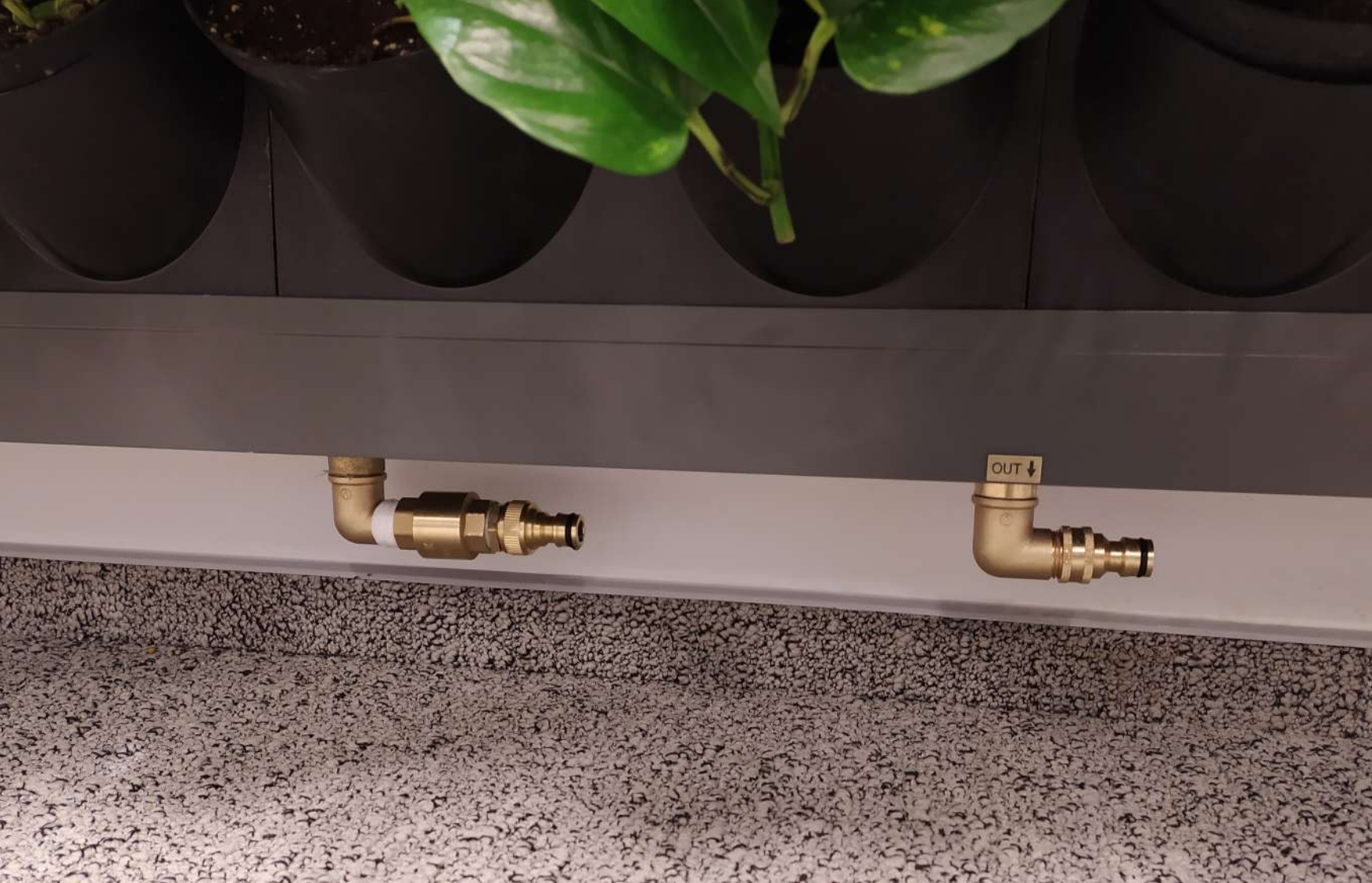
WATER FILLING STATION
